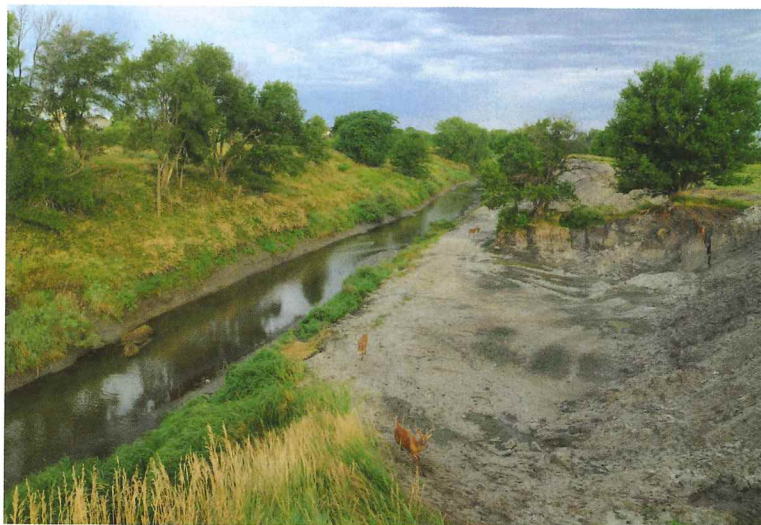
Along Little Salt Creek, excavating and re-shaping a bank to access saline soils and allow for water inundation is the first step in the process.
