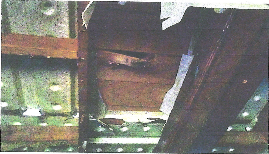
2. Roof Decking Damages near Bay Window – Living Room.
