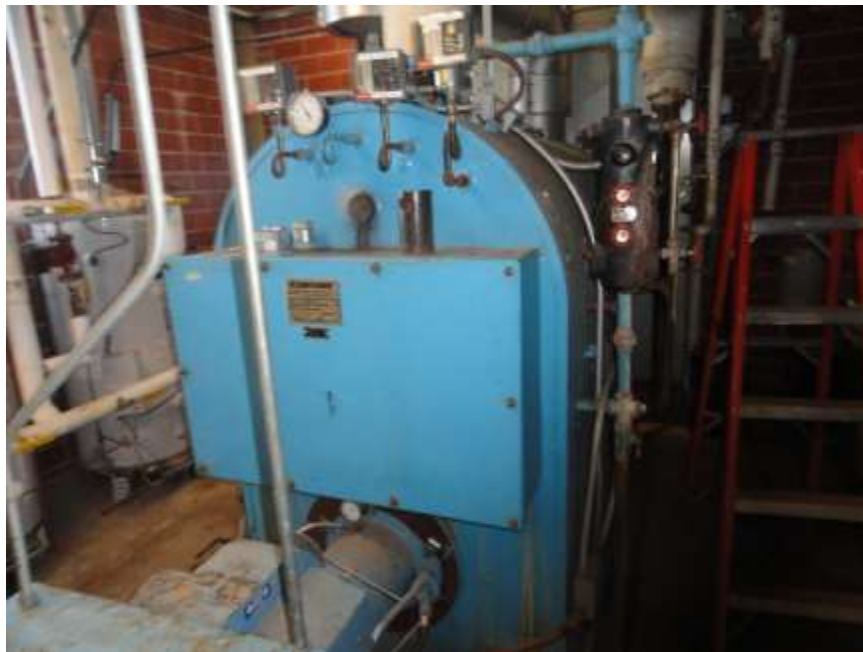
SUBJECT PHOTOGRAPH: SHOWING PENTHOUSE MECHANICAL AREA. SHOWING MECHANICAL ROOM FINISH.
