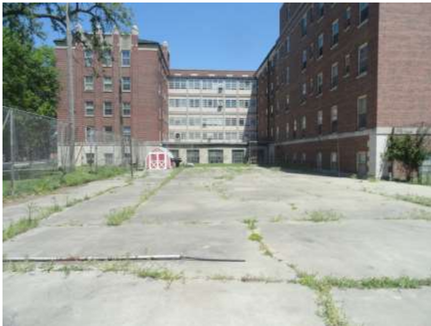
SITE PHOTOGRAPH: LOOKING NORTH ACROSS CENTRAL PORTION OF SUBJECT SITE. SHOWING CONCRETE PAVING IN CENTRAL PORTION OF SUBJECT SITE.
