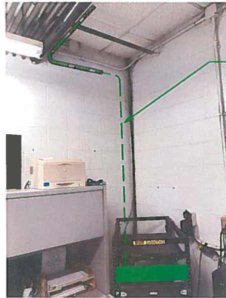
12 FIBER PIGTAIL PULLED THROUGH CUSTOMER OWNED CONDUIT.
