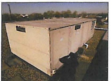
1996 rooftop air handler
