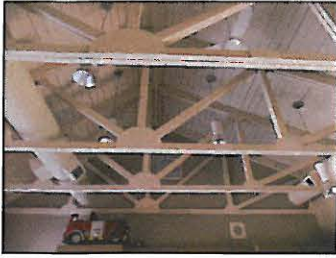
Lighting at Fire/Med #4
