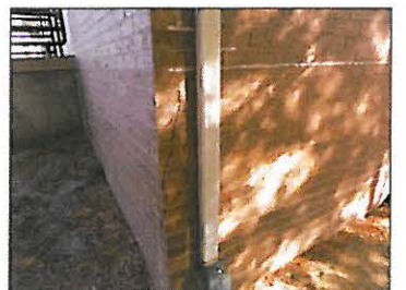
Cracks in bricks
