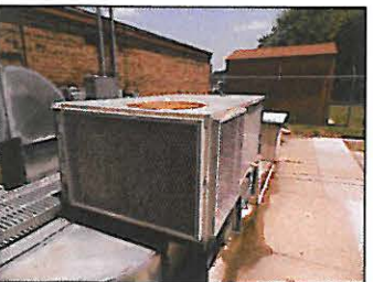
Solid Waste HVAC Unit
