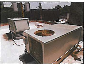
Community Building RTUs
