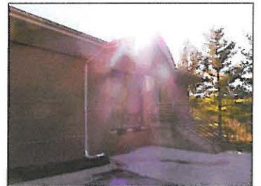
Undersized gutters and downspouts
