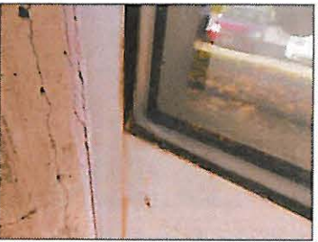
Deteriorating window seals
