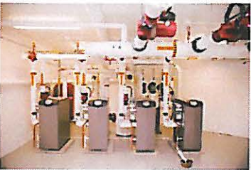
Example High Efficiency Hot Water Plant
