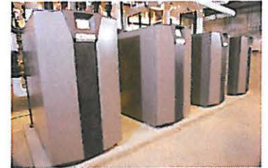
Condensing Boiler Plant
