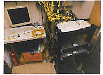
Server Closet at Vehicle Maintenance Garage Office
