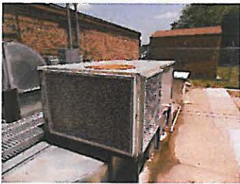
Existing Packaged Unit (2001) at Solid Waste Office
