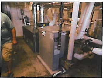
Boiler at Carnegie Building
