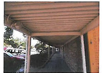
Parking Lot #3 Canopy Lighting and Conduit To Be Replaced
