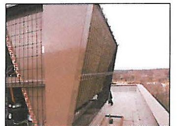
New chiller on roof
