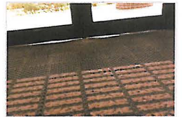
Visible Gap Under Exterior Doors at The Sports Pavilion
