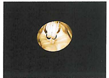
Fluorescent can fixture
