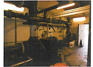
Pool Recirculation Pump
