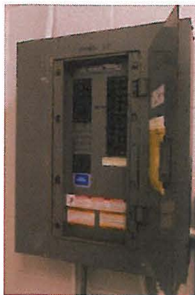
Panelboard with Corrosion
