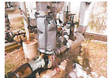
Pump Station at Venture Park Holding tank
