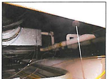
VAV box and HW piping
