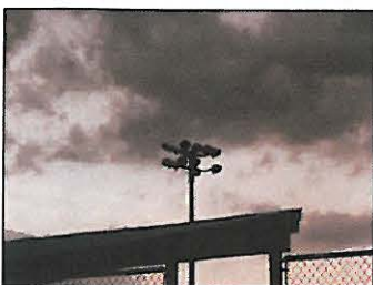
Existing sports field lighting
