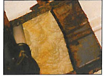
IAC rust from poor ventilation
