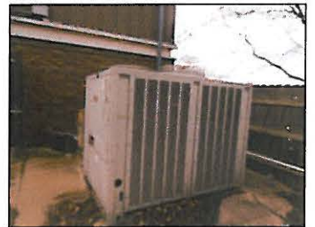
Holcom Center cooling unit
