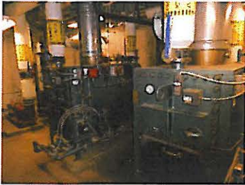
Existing Atmospheric Boilers
