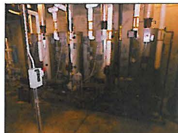
Heating water boilers
