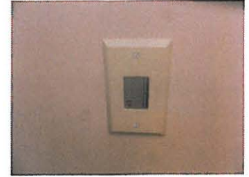
Digital HVAC controls at FS#5
