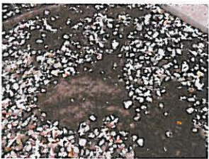
Roof deterioration at FS#3
