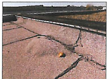
Bubbling on roof
