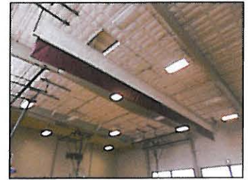
Holcom Center high-bay lighting
