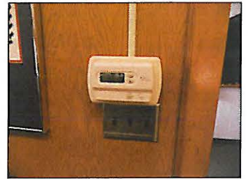
Traditional thermostat at Fire/Med #3
