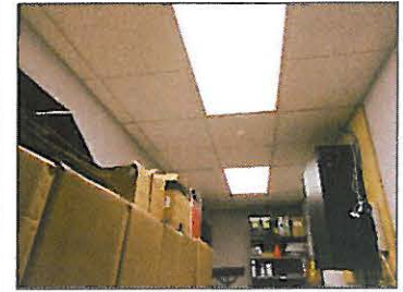
Existing fluorescent lighting
