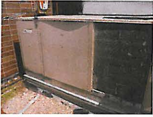
Older RTU at FS#3
