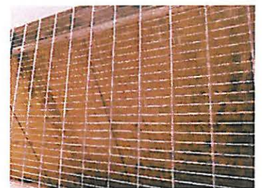
Dirty Condenser Coils
