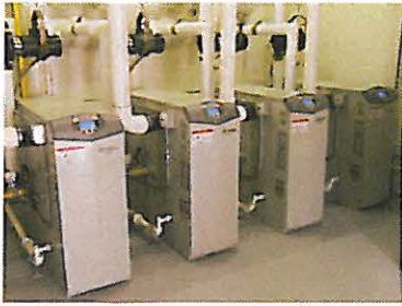
High efficiency condensing hot water boiler plant
