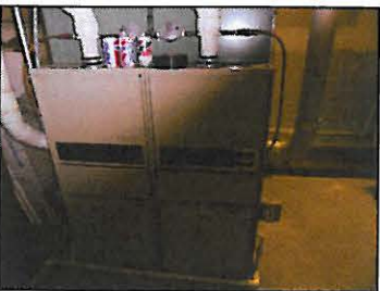
Older furnaces and cooling coils
