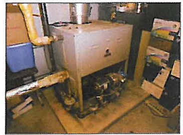
1993 hot water boiler
