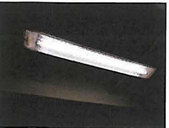
Riverfront garage T5 lighting
