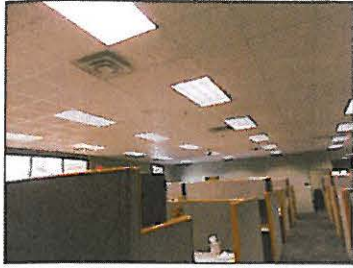
Fluorescent lighting in the office area
