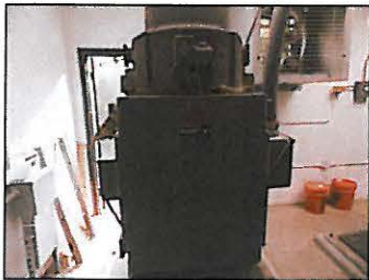
Pump #1 at North Lawrence Pump Station
