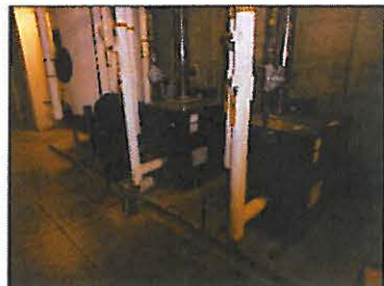
Domestic water heaters
