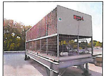
Arts Center Chiller
