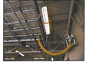
Highbay fluorescent lighting at Fire/Med #2
