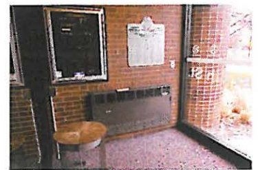
Electric Cabinet Heater at Main Entry
