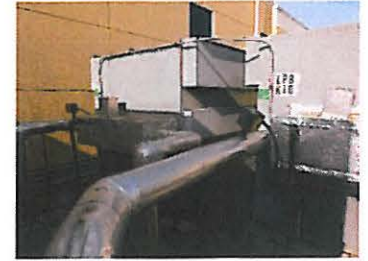
Existing Pool Boilers
