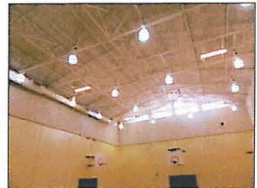
Existing metal halide luminaires in gymnasium
