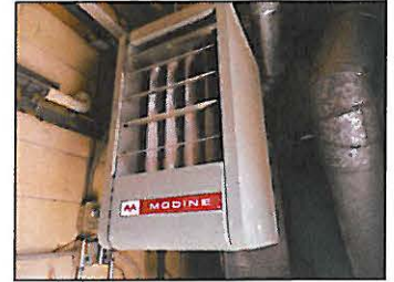
Gas-fired unit heater
