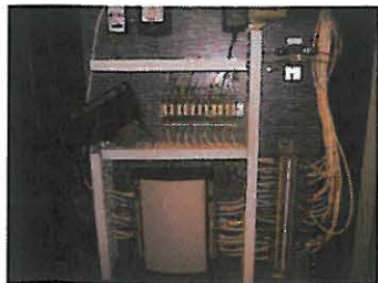
Digital HVAC controls at FS#4
