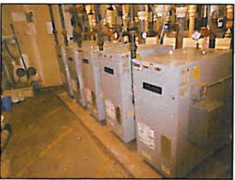
Existing building boilers
