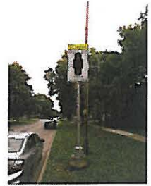
Existing School Zone Beacon Powered by Electric Utility
