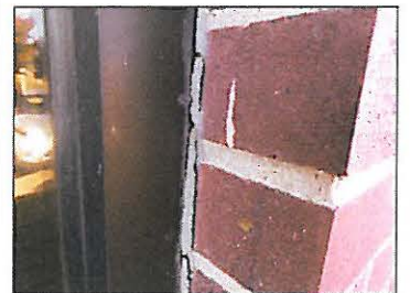
Deteriorating window seals
