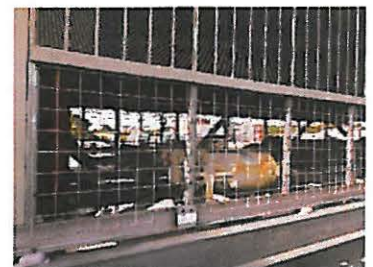
Existing Helical Rotary Screw Compressor
