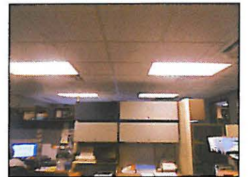
Existing T8 Lighting
