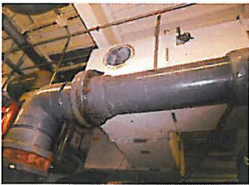
Decommissioned Exhaust Duct
