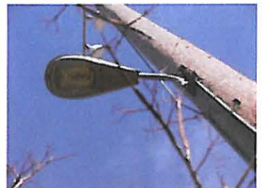
Walkway Area Light
