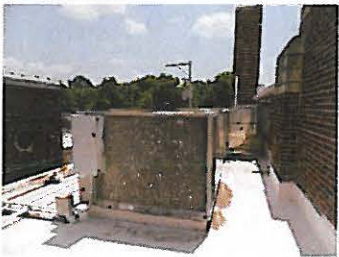
Rooftop Hail Damage
