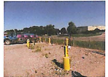
Block Heater Receptacles on Bollards
