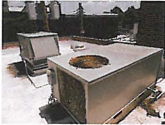
Existing Packaged Unit (1993)
