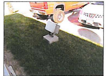
Existing metal halide flood lights
