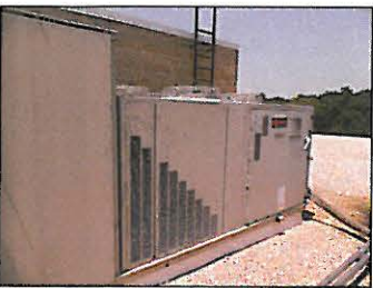
Packaged rooftop unit
