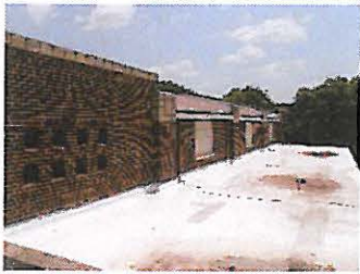
Rubber Membrane Roof
