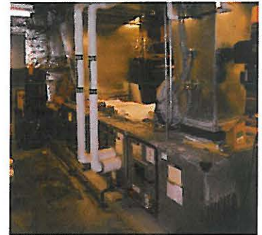
Single Zone Constant Volume Air Handling Unit
