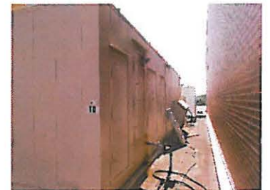
Existing Packaged Dehumidification Unit
