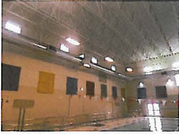
Existing Supply Ductwork in Lap Pool and High Return
