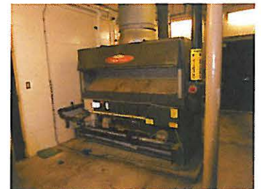
Pool Water Heater
