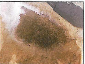
Standing water on roof
