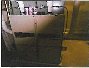
Older furnaces and cooling coils
