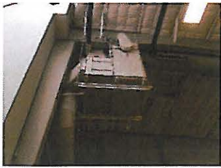
Gymnasium Air Handler
