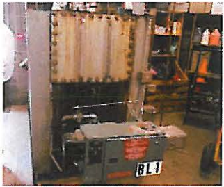
Aging AJAX Boiler
