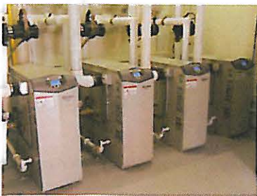
High efficiency condensing hot water boiler plant
