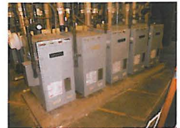
Failing Twenty Year-Old Condensing Boilers in Community Health Building
