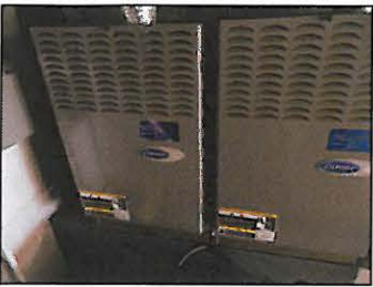
Fire & Rescue Training Center HVAC
