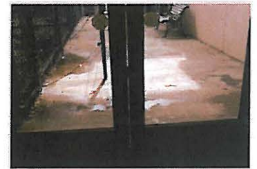
Gap Between Doors Due to Worn Weather Stripping at Prairie Park Nature Center
