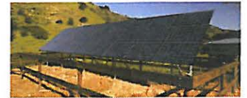
Remote Photovoltaic Array Used for Solar-Powered Water Pumping
