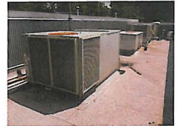
Older RTU at FS#2
