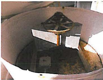
Decommissioned Exhaust Fan
