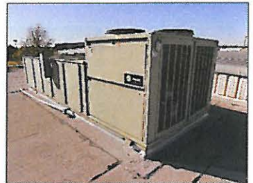
1986 DX/Gas VAV rooftop unit
