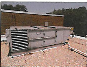
Outdated rooftop unit
