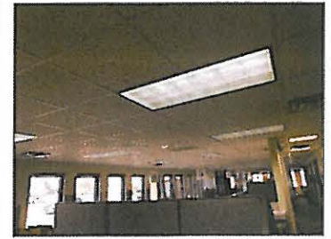
Existing fluorescent lighting
