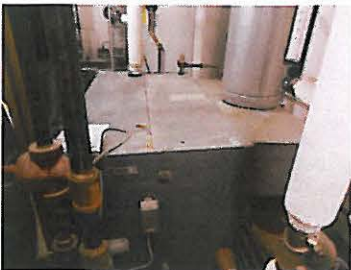
Existing Heating Water Boiler
