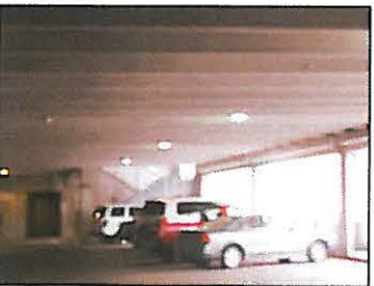
Metal halide lighting at New Hampshire parking garage
