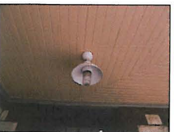
Exterior Depot Lighting
