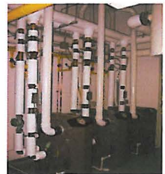
Central Hot Water Plant
