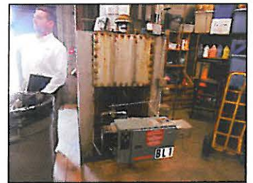
Holcom Center boiler
