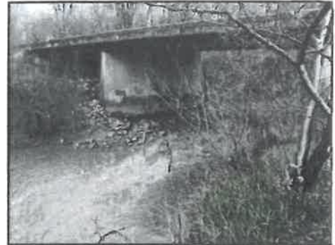
Figure 7-10: Knickpoint and Exposed Bridge Piers
